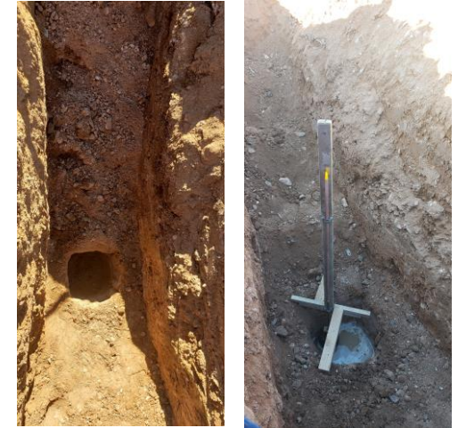
Figure 5: Typical test pit after excavation (right) and a test pit with ongoing infiltration test (left).
